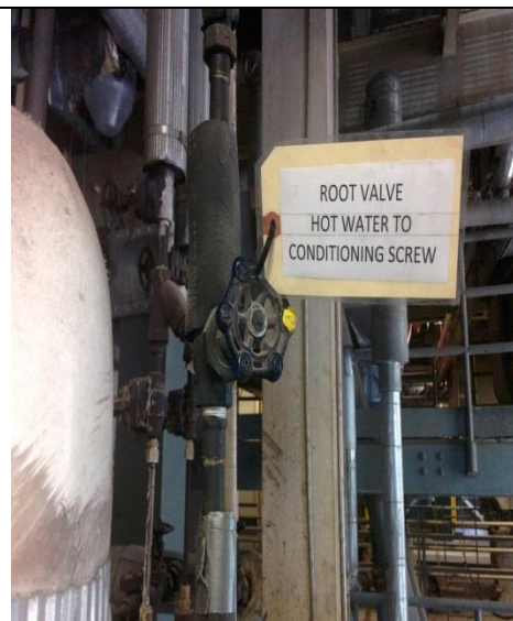
Figure 30 A parallel boiler hot process water injection is sent to fly ash
