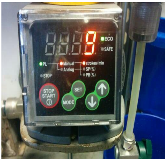
Figure 33 Conducting pump trial settings
